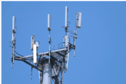
Wireless Base Station
